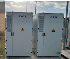
09. Battery Rack (Quelle: SMA Solar Technology)
